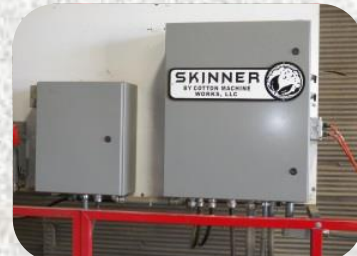
PLC & VFD DRIVE PANELS
