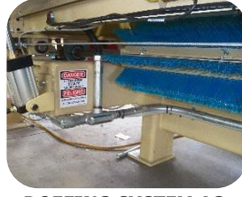
DOFFING SYSTEM AS VIEWED FROM BELOW WITH SAFETY CABLE SWITCH
